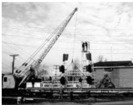
Cantilevers were added to signals at the Belt’s Columbus Avenue crossing at Southwest Highway.
