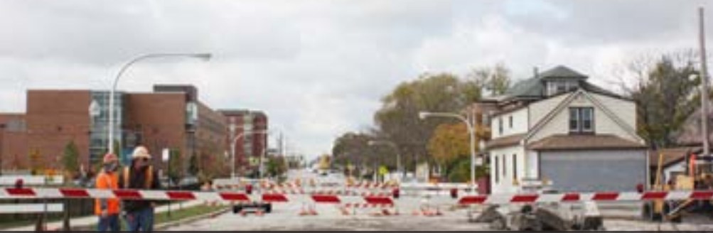
Employees work on a new grade crossing at 67th Street near Mariano Azuela Elementary School.
